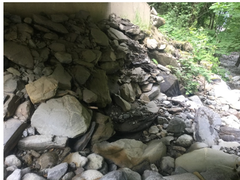
Left bank riprap scour
