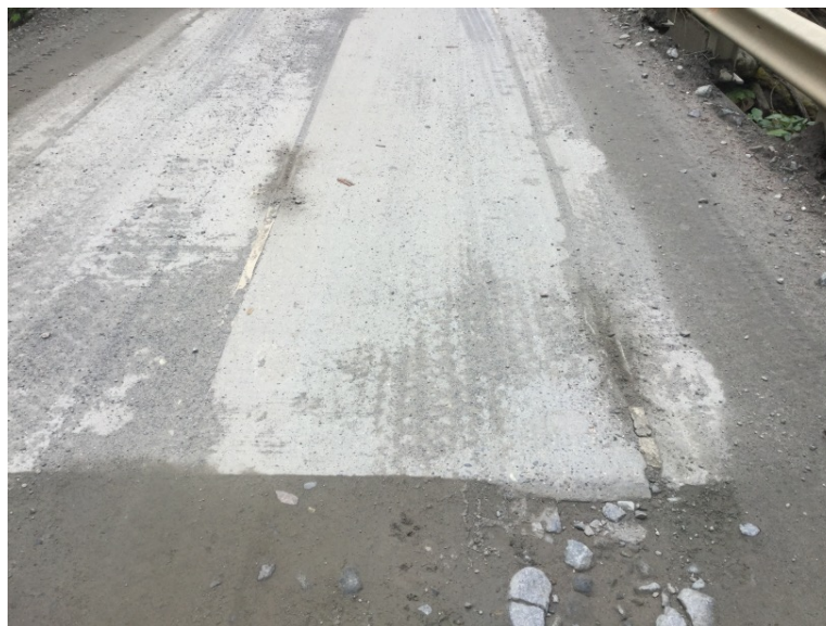
Paraseal joints have failed
