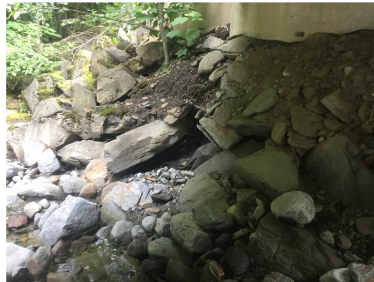
Right bank riprap scour
