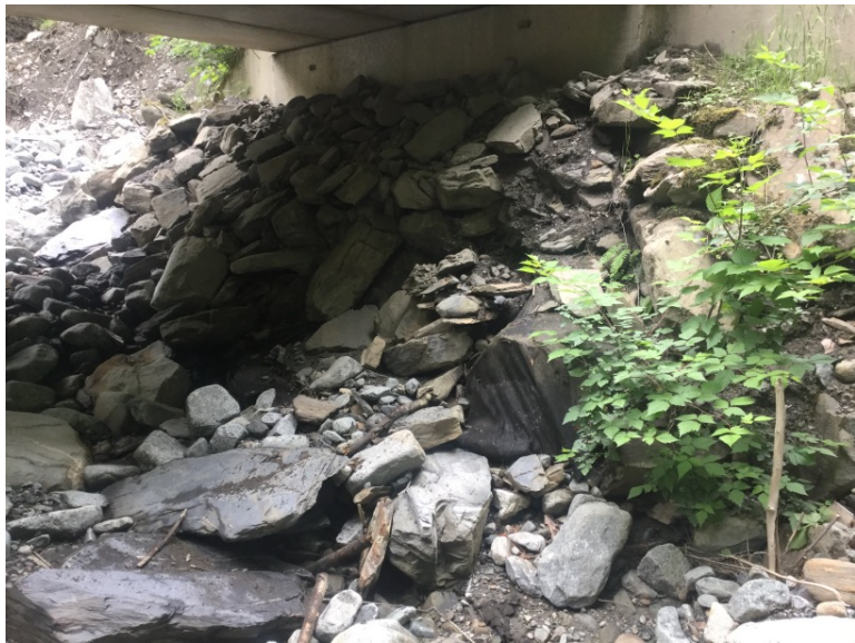
Downstream left bank scour
